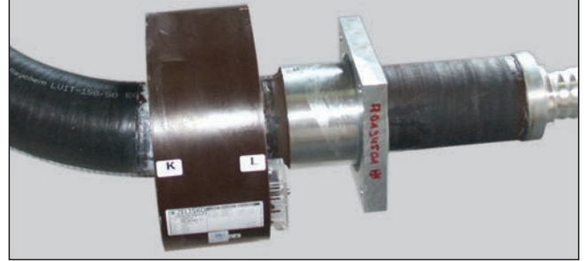
Fig. 1: Instrument Transformer Integrated
